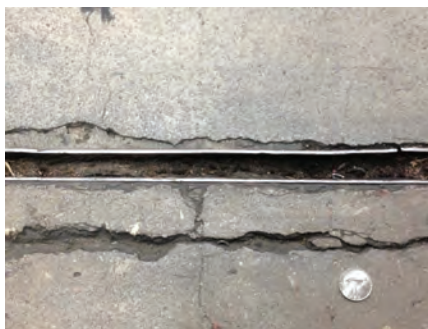
Figure 1a: A typical construction joint opening in a ground-bearing concrete slab. The joint gap width is a function of concrete drying shrinkage.
