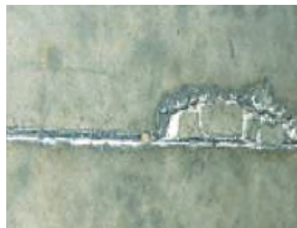
Figure 1b: A typical saw-cut induced contraction joint. Saw-cut joints allow curling to take place and introduce a point of weakness where damage is localised requiring repair.
