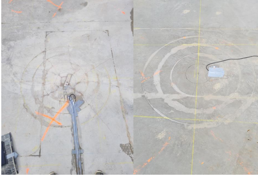
Fig. 4. Comparison of crack patterns in place of maximum negative bending moment after LL3, left – SFRC, right – SFRSSC.
