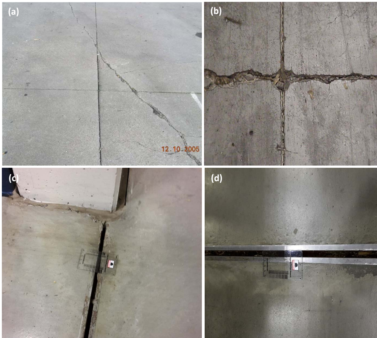
Figure 1: Typical issues with industrial concrete floors resulting from the drying shrinkage of concrete.
